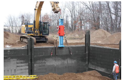
Step 9. Depending upon depth of system, rigging may have to be choked up or moved to higher connection point on the Panel Pusher. Repeat steps 6 - 9 as needed to remove system.
