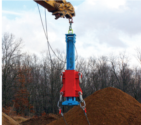
Step 5. With hoses connected, attach rigging to lower connection, and move to Slide Rail System.
